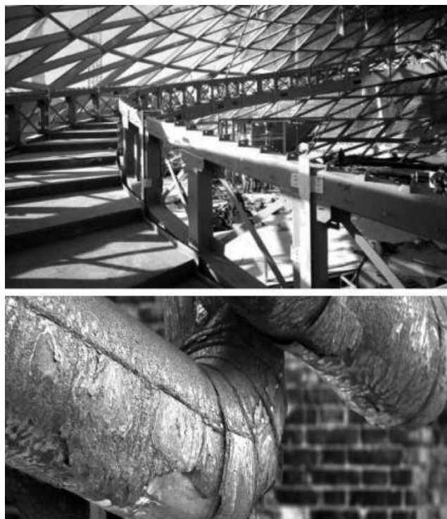
Figure-1. Corrosion affecting the metal structure
