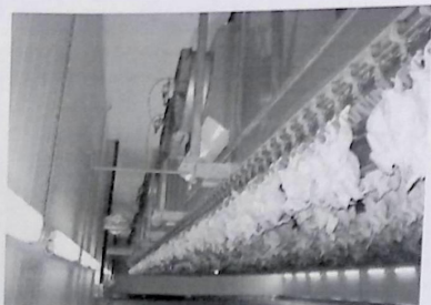
FIGURE 20.3 Continuous air-chilling system for whole poultry.
