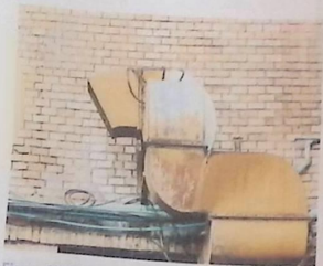
Figure 13.13(a) Local exhaust ventilation systems can quickly corrode and need regular maintenance of fans and filters
