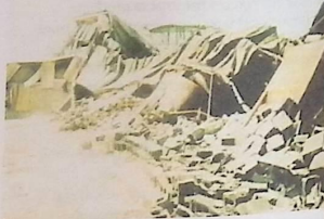
Figure 12.15 Steel structures can collapse in the event of a fire
