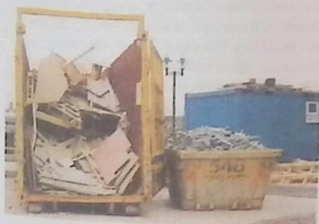
Figure 13.21 A designated waste collection area with two types of skip commonly used for waste collection. Heavy materials would be transported in the smaller skip. Sizes of skip range from about 4 cu metres (small skip shown) to about 35 cu metres (large skip shown)
