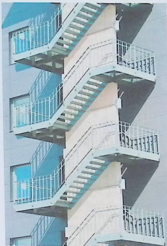
Figure 12.24 External fire escape from a multi-story building. Extreme caution needed in winter and enclosure of staircase would be preferred for the UK climate
