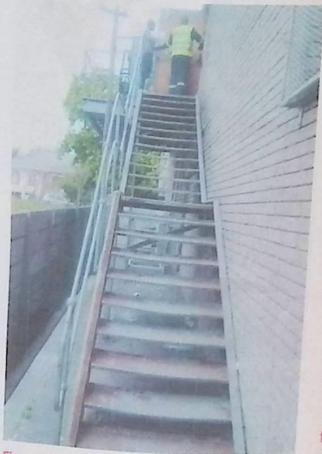
Figure 12.25 Fire escape route outside building
