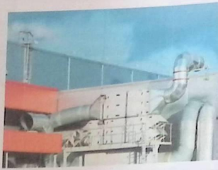
Figure 13.13(b) Large roof level system with access platforms for maintenance of the filters and fans
