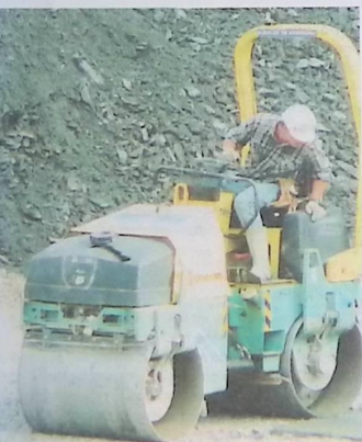
Figure 14.7 (a) Vibrating roller with risk of whole-body vibration
