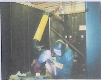
Figure 13.12 (a) A LEV system; (b) welding with an adjustable LEV system to remove dust and fumes
